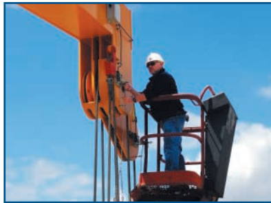
Even the most challenging jobs are performed safely and skillfully by Appleton Marine's field engineers.
