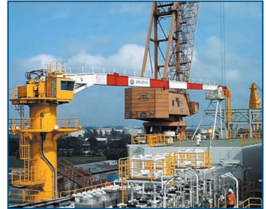
Offshore Maintenance Crane
